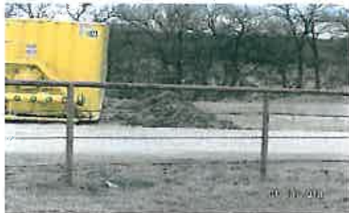
Hydrocarbon impacted soil removed from tank spill
